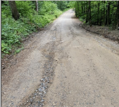
Erosion along Kaulback Road.
