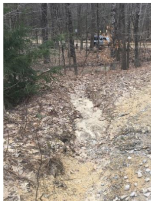
Site 10. Roxbury Road
