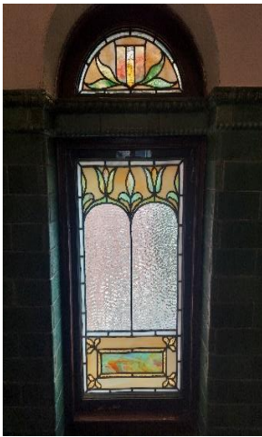
3. Stained glass before it was removed from the rotted window casing.
